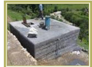
CWR & chlorinator of a W/S scheme
